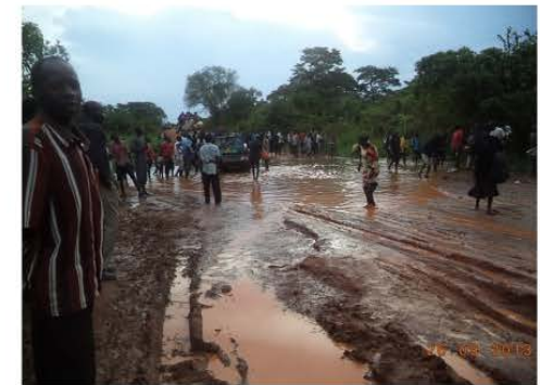
Effects of floods on roads and bridges
